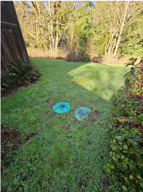
Photo 3 (Map Photo ID 304): Septic tanks on the west side of the house—the caps look new.
