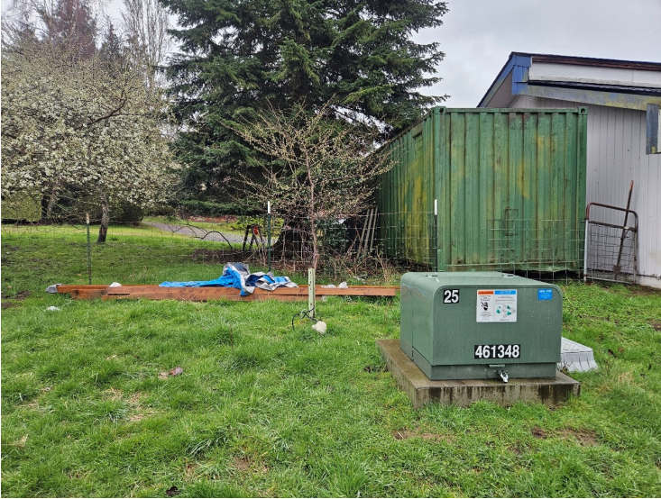
Photo 13 (Map Photo ID 288): Transformer box on the north side of the garage.
