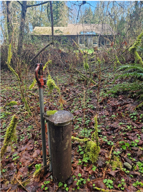
Photo 7 (Map Photo ID 314): Drilled well head and spigot south of the residence. No well tag was present. Just to the south of the well head there is a small wetland.
