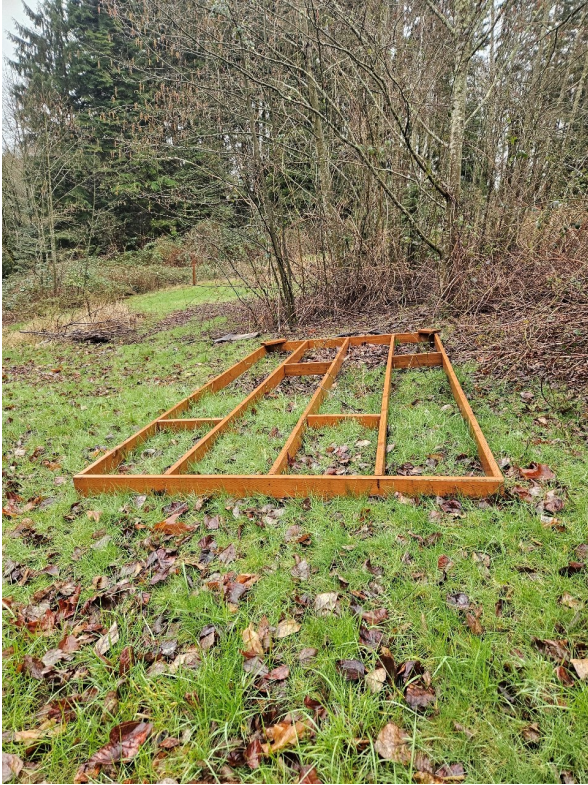
Photo 18 (Map Photo ID 297): Framing for a structure located in the central portion of the property.
