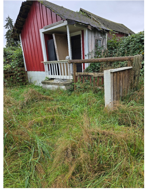
Photo 8 (Map Photo ID 165): An old storage shed near the southern edge of the property. This likely needs to be torn down, as its highly compromised.
