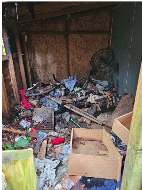
Photos 4 (Map Photo ID 216 & 217): Inside the storage sheds from Photo (4). They were filled with junk, chemicals, clothes, etc. Staff were unable to investigate inside the sheds due to their condition.
