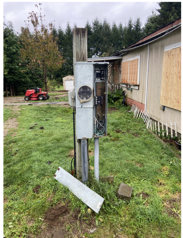
Photo 19 (Map Photo ID 137): Electric/utility pole on the south side of the mobile home.
