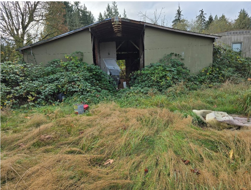
Photos 7 (Map Photo ID 207): An old barn filled with tires, carpets, bath tubs, chemicals, and various junk (both within and around). Located on the southern portion of the parcel.
