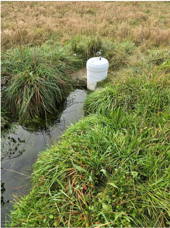
Photos 8 (Map Photo ID 196): Well which services all parcels part of the Schultz Clan Property. A pipe runs from here, north to the new Well House. Previous tenants had broken the pipe, creating a serious leak, as surface water can be seen pooled around the wellhead.
