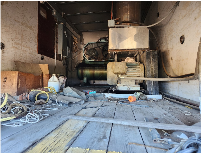
Photo 10: Inside the yellow, semi-permanent structure featured in Photo (6). This structure houses an air compressor that feeds airlines throughout the main shop and secondary shop on the property. Map Photo ID: 55.1
