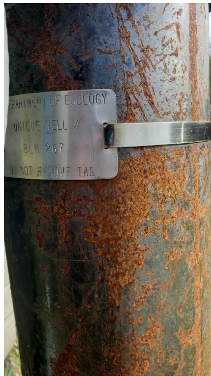
Photos 2 & 3: The drilled well and pressure tank for the property. This infrastructure is located just to the south of the residence on the property. The well infrastructure appears to be functional, despite the shoddy appearance.
