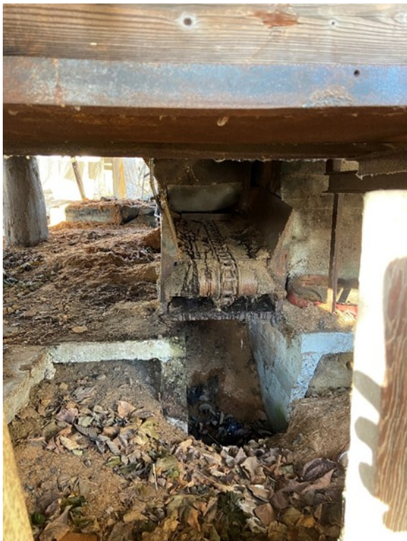
Photo 15: Chain return trough for the conveyor belt seen above. Upgrades have been made to the mill apparatus that have made the trough irrelevant. Before, the trough was approximately 3-4 feet deep. Simple soil sampling confirmed no obvious signs of hydrocarbon contamination.
