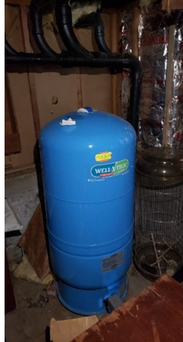
Photo 5 and 6: Inside the room under the deck stairs which houses the well/water infrastructure. Everything seems new and up-to-date. This services both dwellings on the property.
