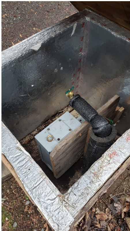
Photo 25: A closer look inside the RV hookups box.
