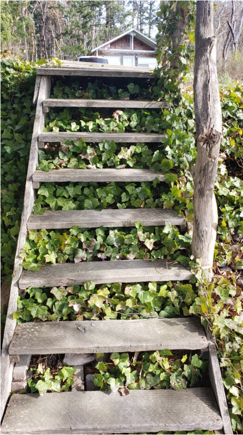
Photo 23: The steps leading down from S Barnum Road—the Vo Residence can be seen in the background. These steps are in disrepair and very rickety and appear to be located on the Vo parcel. Photo taken looking north.
