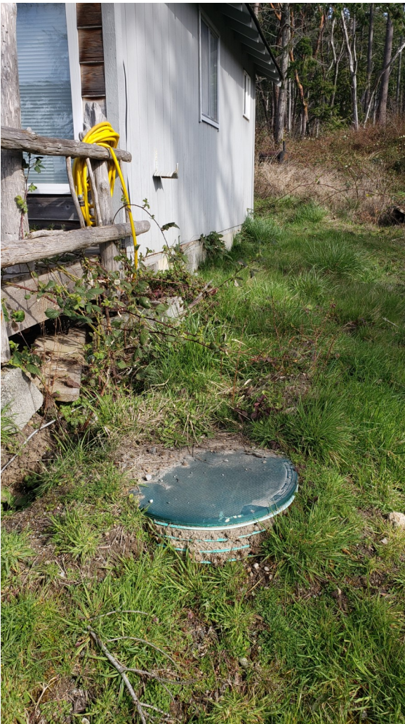
Photo 20: The septic tank on the property, just to the east of the residence. Photo taken looking north.
