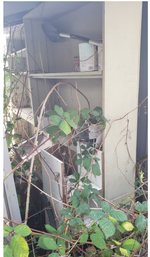
Photo 9: The backside (north) of the outbuilding from Photo (6). An assortment of used paint cans and other household materials were found. These items should be properly disposed of prior to closing.
