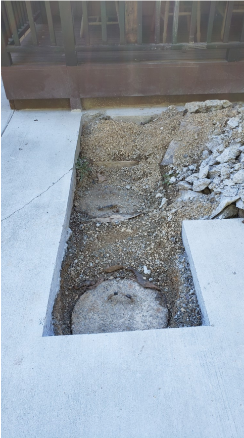
Photo 10: Septic tank access points, just off the deck of the main residence. The contractor which laid the concrete accidentally covered this access points.
