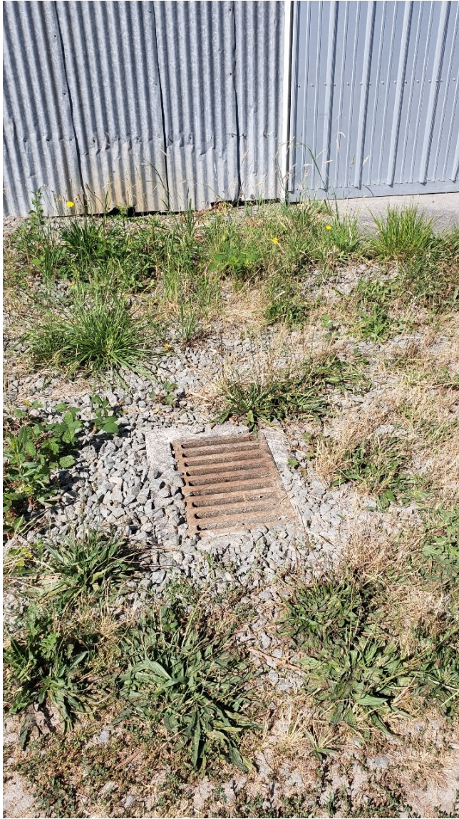
Photo 44: A drain outside the north shop (in the parking area). Staff were unsure if this discharged into a French Drain system, an Underground Storage Tank, or piped to another location.
