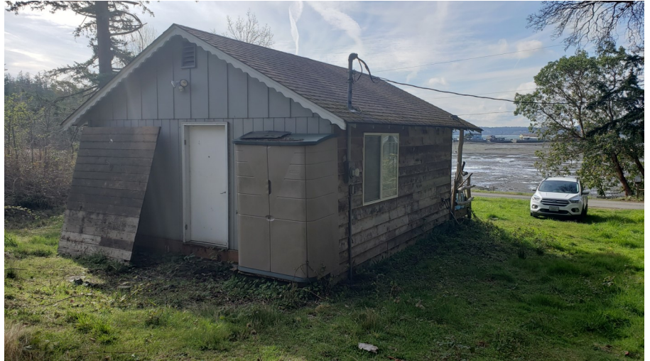
Photo 5: The northern side of the residence. Triangle cove can be seen to the south.
