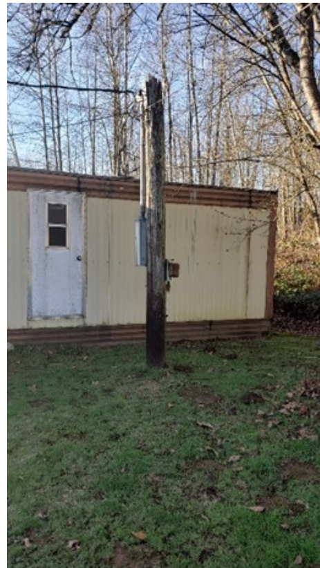
Photo 49: Rotting power pole, next to the mobile on the eastern side of the building.
