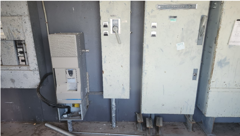
Photo 42: Electrical equipment inside the pump house featured in Photo (40). Map Photo ID: 99.1
