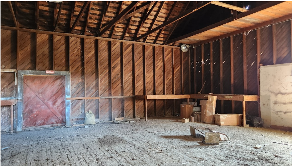
Photo 18: Inside the historic barn. Old desks, equipment, and refuse were found. Staff did not locate any HAZMAT. Map Photo ID: 35
