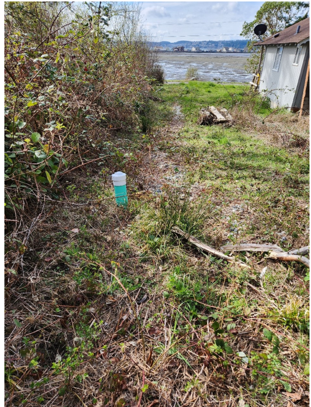
Photo 18: Looking down the eastern property line, a pipe presumably involved in the septic system was located. Additionally, river rock has been used as fill for a trench that was dug leading away from this pipe. Photo taken looking south.
