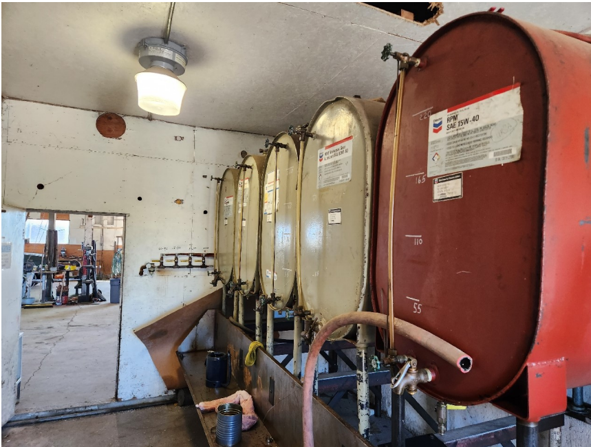
Photo 5: A storage room for various motor oils and hydraulic fluids. Each tank holds approximately 275 gallons. The floor was gently sloped to the west and with evidence of spilled oils and fluids. However, staff investigated soils on the western wall of this room (from the outside) and did not find any surface contamination. Map Photo ID: 45.2
