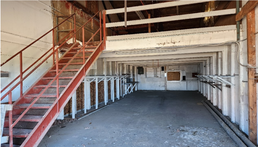
Photo 31: Inside the second shop, a staircase leads to an upstairs storage area. Picture taken in the western half of the second shop. Map Photo ID: 68.1
