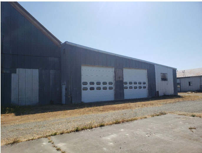
Photo 12. The western side of the automotive/equipment repair section of the main shop. Photo taken looking east. Map Photo ID: 52.
