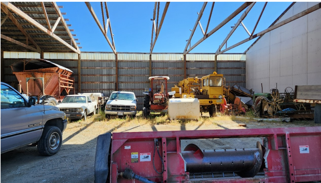
Photo 26: A section of the pole barn which lost its roof. More equipment and oil stained gravels were found here. Map Photo ID: 83.1
